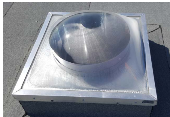
Figure 7. Trapped Condensation in the Solar Tube
