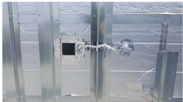
Figure 5. External Heat Flux, Temperature and Pressure Installation
