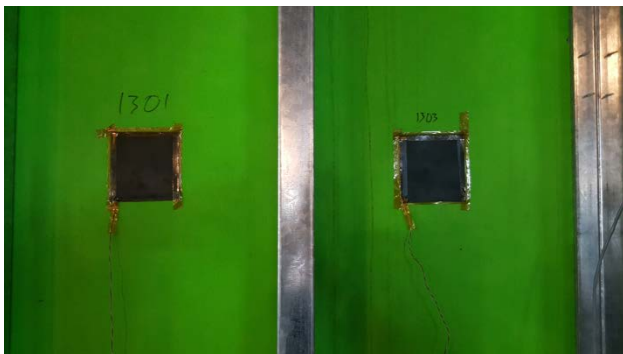
Figure 4. Interior Heat Flux Sensor Installation
